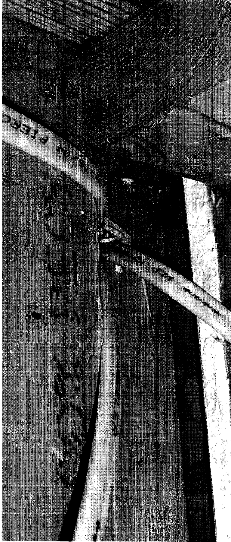
Photograph of the labeling on the back of the sheetrock in the attic.
