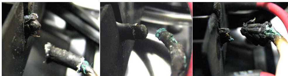
Figure 5-6. Melted connections at the heating element (three additional incident samples)
